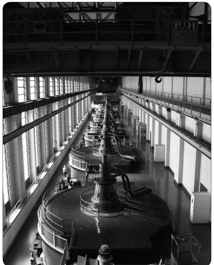
Photo of Safe Harbor Water Power Corporation on the Lower Susquehanna River in Pennsylvania.
