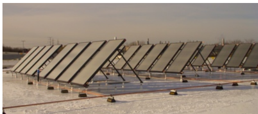
Many people think of solar water heating systems as a couple of panels on the roof of a home, but there are many large systems like this one that provide hot water to college dorms, factories, and other large facilities. Photo courtesy of Johnson Controls, Inc.
