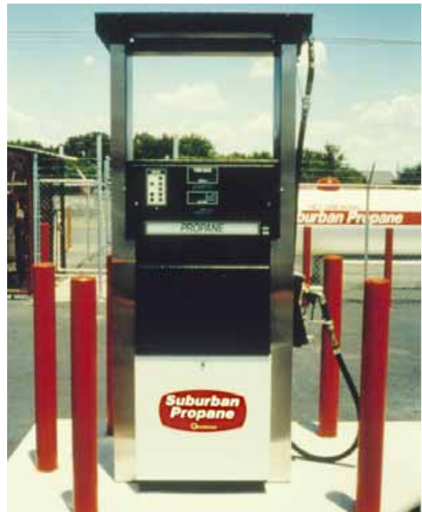
Propane filling station.
