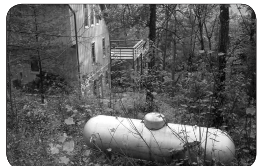
Propane is stored in a large tank. It is used to provide energy for heating, cooking, and drying clothes.
