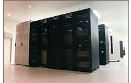
Data centers help the Internet run smoothly, but use large amounts of energy. Photo Credit: DOE
